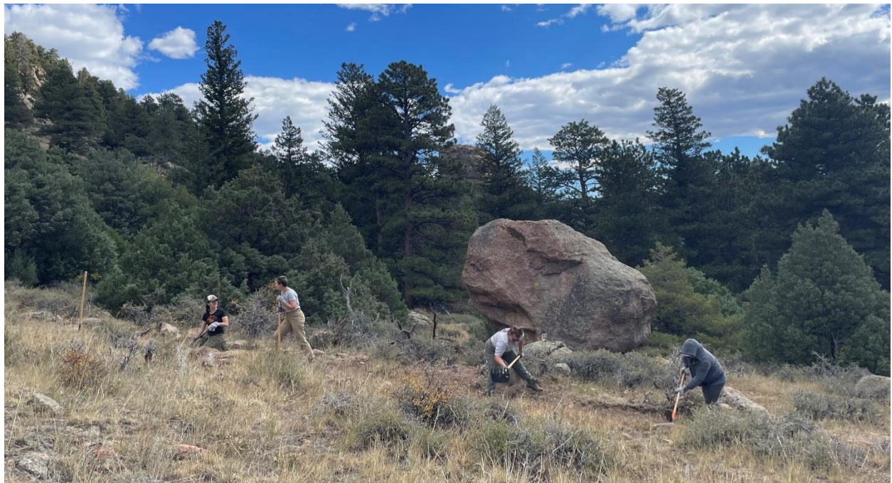
The crew hard at work widening a section of trail. The large boulder in the background is called the “Equalizer” boulder and is another climbing destination in the Thumb Open Space.
