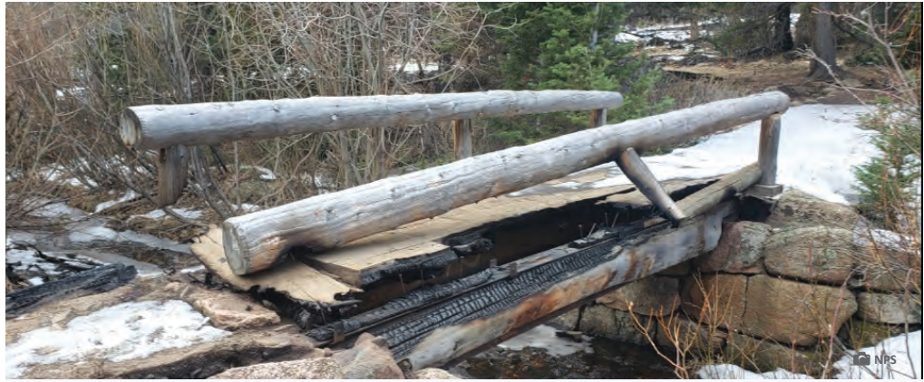
Mill Creek Trail bridge burned by the East Troublesome Fire that is slated for repairs
