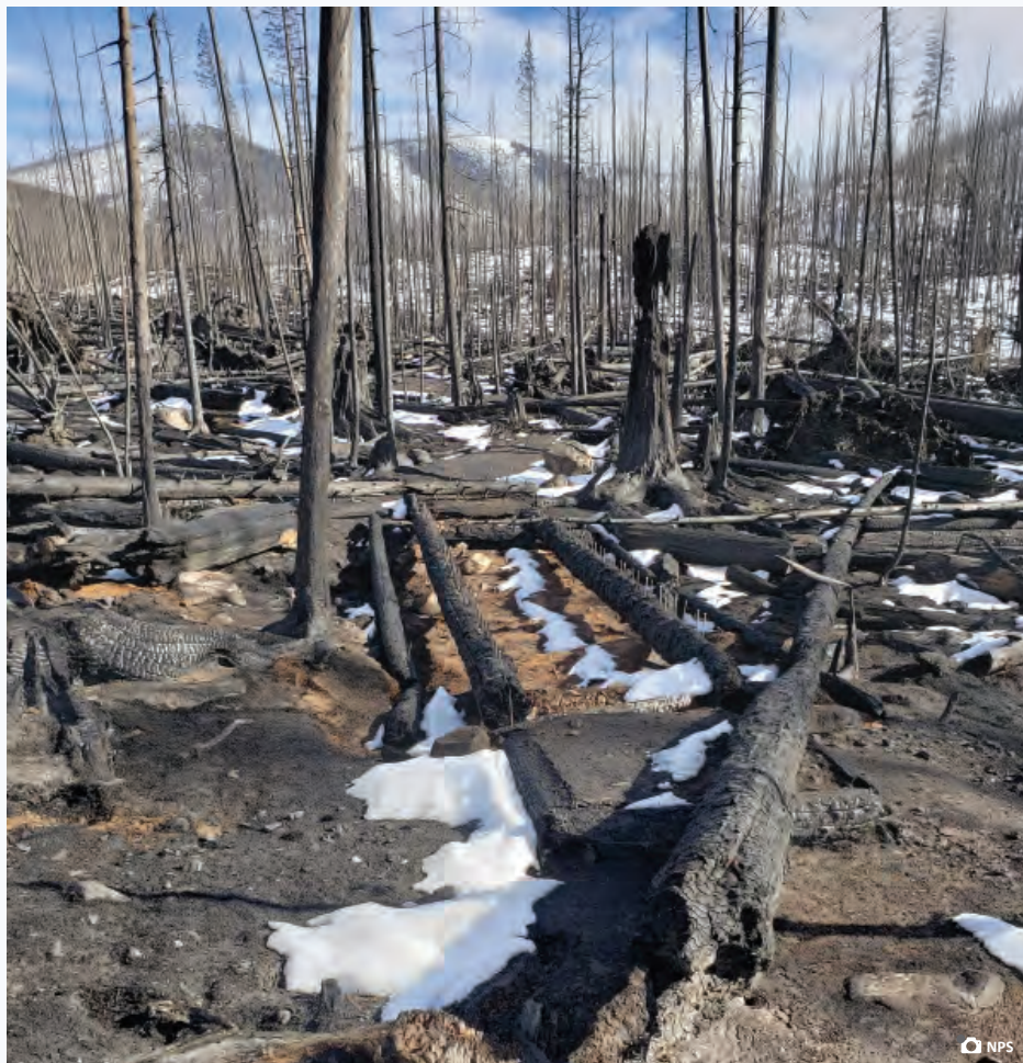
Burned Green Mountain Trail Bridge on the park's west side
