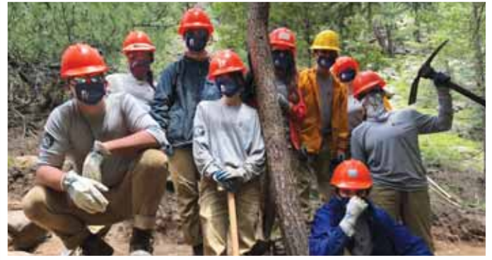
The Boulder Crew completed a rock wall project to help fortify the edge of the trail along the downhill slope to prevent erosion.
