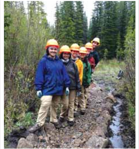
High School Leadership crew proudly presenting the new turnpike they helped build.
