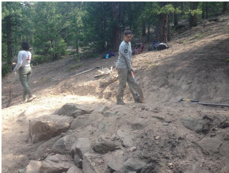
Estes Crew members work to construct a switchback on the Aspen Brook Trail, which was destroyed by the 2013 Colorado floods.
