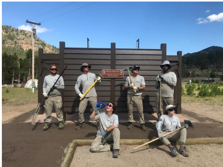
Moraine Crew works to establish a trail to their recently constructed solar shower station at Glacier Basin Campground.
