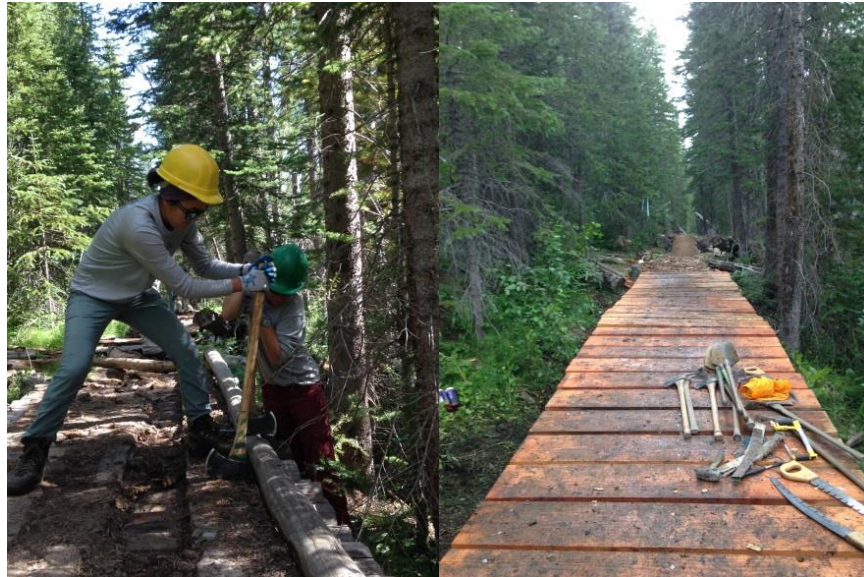
Photos: Crews working to deconstruct and replace board on McIntyre Trail boardwalk.
