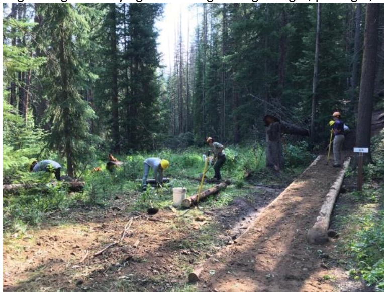
Photo: The crew with the nearly completed turnpike on Ice Hill Trail.
