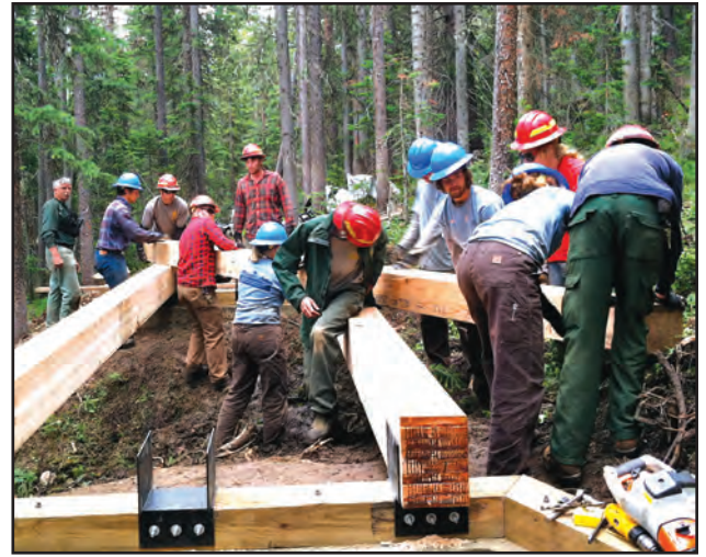
The Shadow Mountain crew working on a major bridge on a west side trail.
