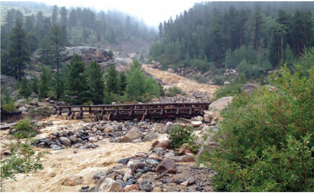
The Roaring River took on epic proportions as it barrelled down the canyon, shouldering boulders aside, damaging the bridge and ripping out part of Endovalley Road before creating a brand new alluvial fan in the meadow.
