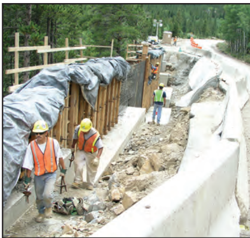
Panels poured and curing, again, for the upper segment of Bear Lake Road in Phase I.
