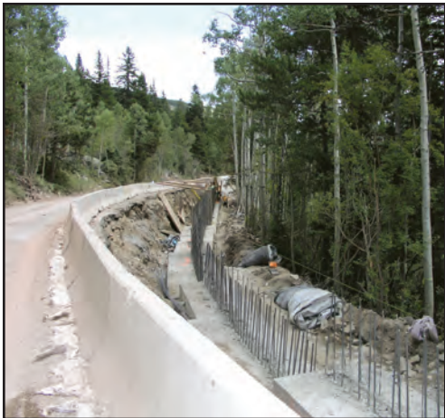
Erecting wall panel forms for the upper segment of Bear Lake Road in Phase I.
