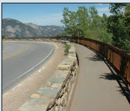
American Recovery and Reinvestment Act funds funded the replacement of the deteriorated boardwalk at Many Parks Curve.
