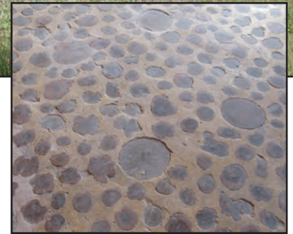
The dining room, which occupies one of the two hexagonal-shaped rooms within the building, has been restored to its original splendor, including the unusual floor which is made of log rounds encased in concrete. Guests of the Onahu Ranch enjoyed home-cooked meals here as part of their Western vacation. In a brochure from the 1950s, hosts Joe and Myrtle Bolder describe the dining room as "large and cheerful and the food is well planned and prepared, served family style in an attractive manner, for outdoor appetites."
