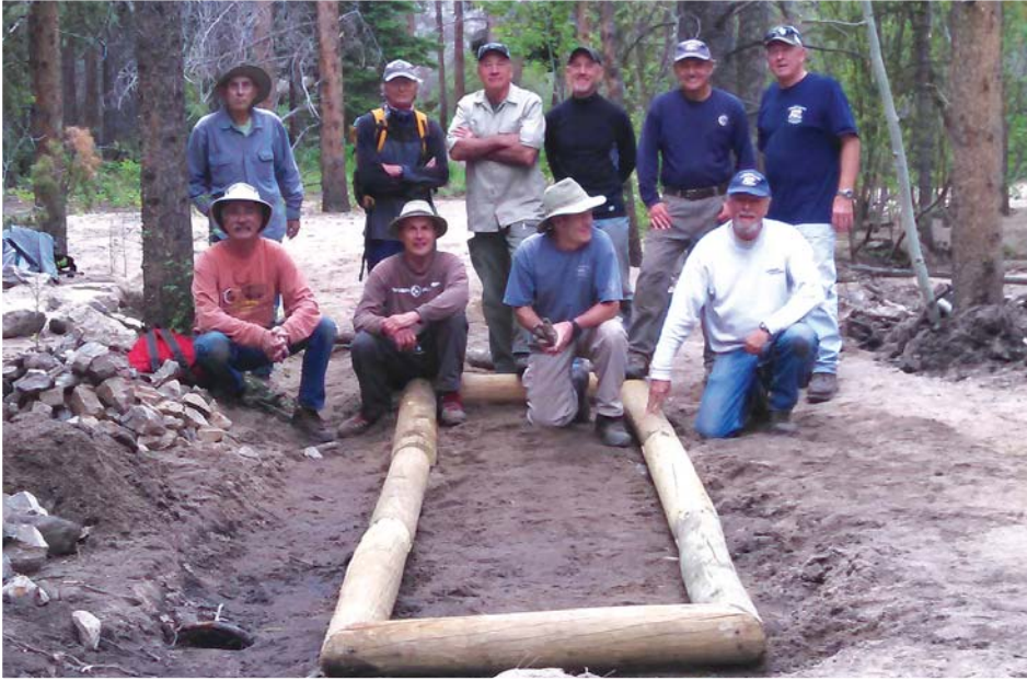
Volunteers with a section of the elevated causeway they were building on the Fern Lake Trail.
