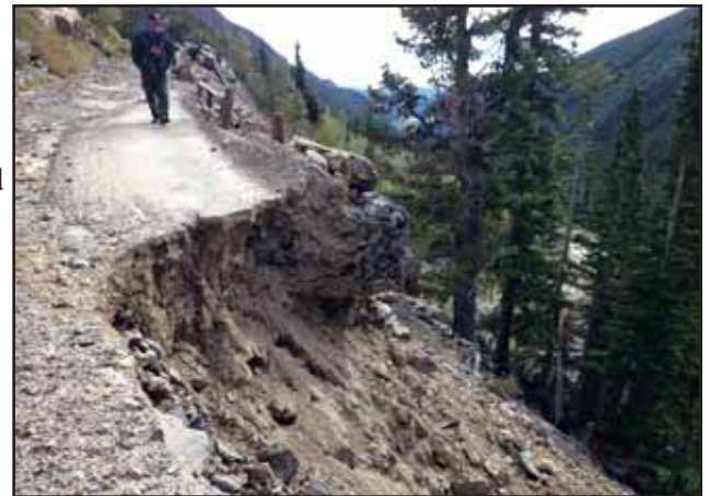
Massive amounts of erosion on Old Fall River Road, among other issues, will close this road for 2014.
